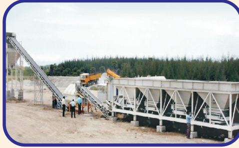
Wet Mix Plant
